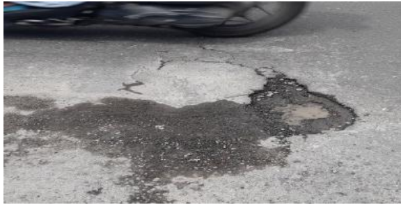
Gambar Kerusakan Retak Slip Sta 1+825 – 1+850
