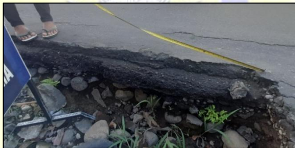
Gambar Kerusakan Penurunan Bahu Jalan Sta 1+800 – 1+825
