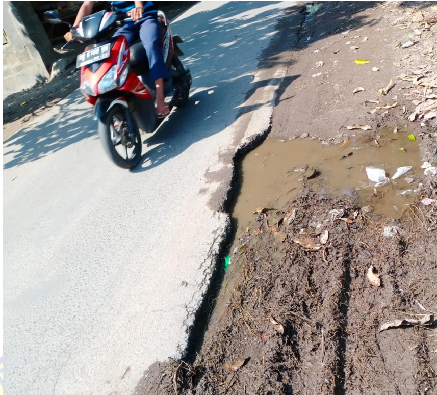
Gambar kerusakan penurunan bahu jalan Sta 2+250 – 2+300
