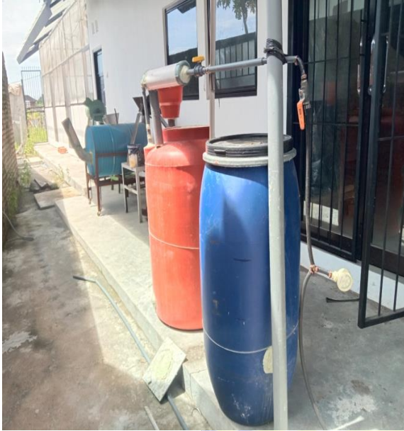
Digester Biogas Portabel
