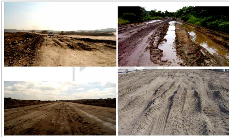
Gambar 2.18 Kerusakan Lendutan ( Rutting ) (Sumber : Report PT.PAMA, 2015)
